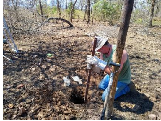
Chris Joubert digging a hole using a metal beam to plant a fence post for one of the bomas that were built. A mechanical auger was available but due to rocks in the soil, the holes had to be dug by hand
